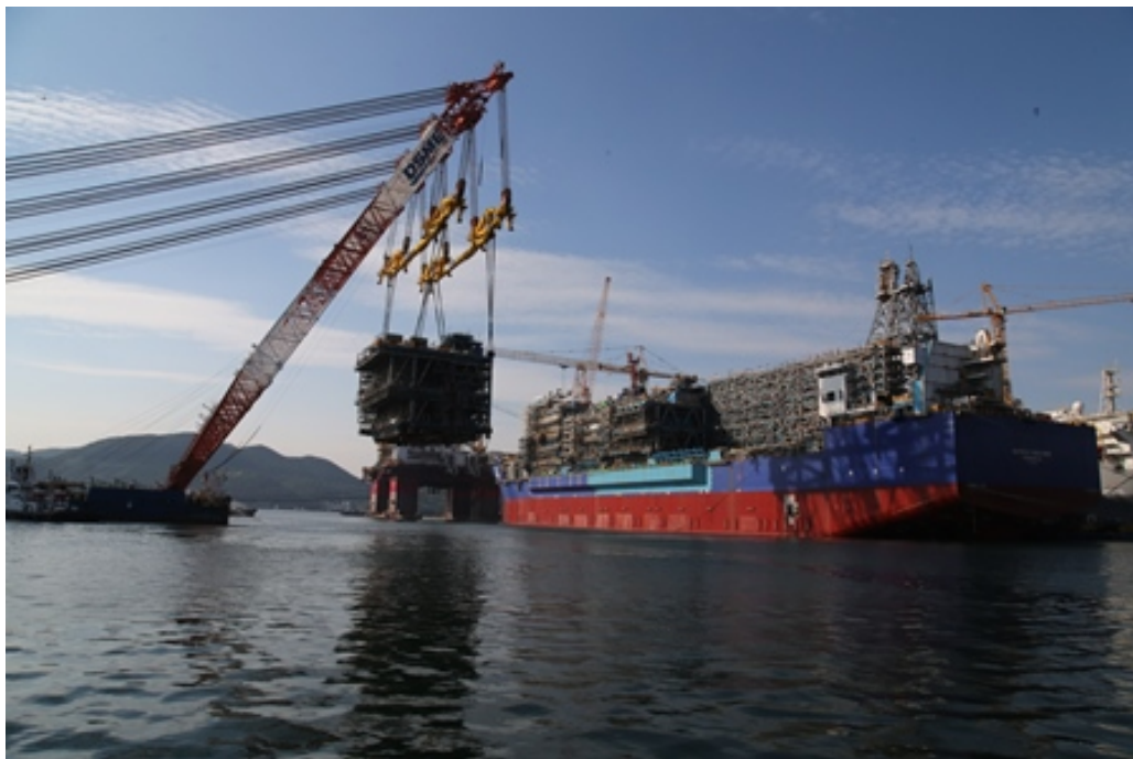
Caption 2: The mono-ethylene glycol injection module successfully lifted and installed onto the hull of the Ichthys LNG Project FPSO in South Korea.
